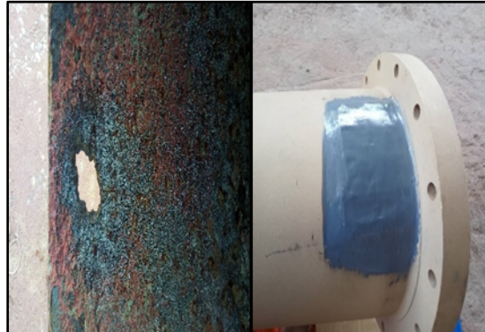
Pipe hole on left and patch section on right.
